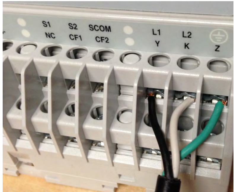
Figure 1 - Temporary Power Connection
